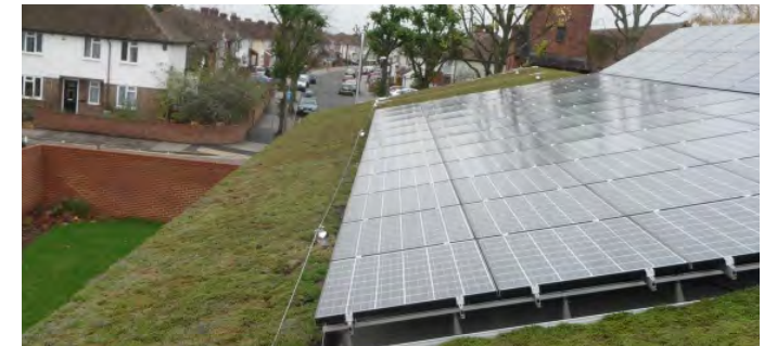
Figure 136: Green roof combined with solar panels.
