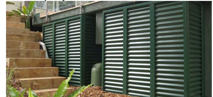
Figure 135: An example of concealed tanks used for rainwater harvesting
